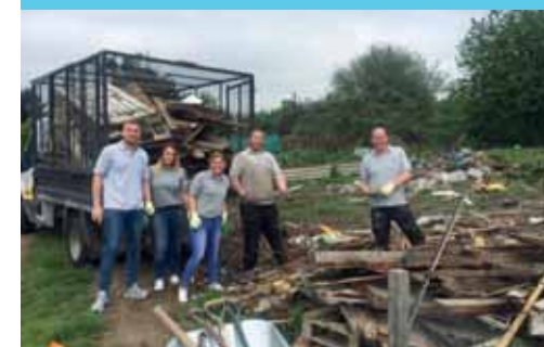
As part of the allotment project our Paragon team helped Walton Charity to clear and prepare a new allotment area ready to be used by the local residents.
