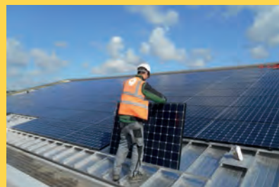
With 750 solar panels, Keynsham Civic Centre can generate 50% of its annual energy requirements.
